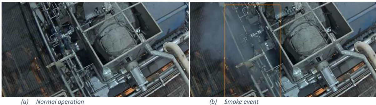
Figure 12. Example of a real incident in machine hall.
