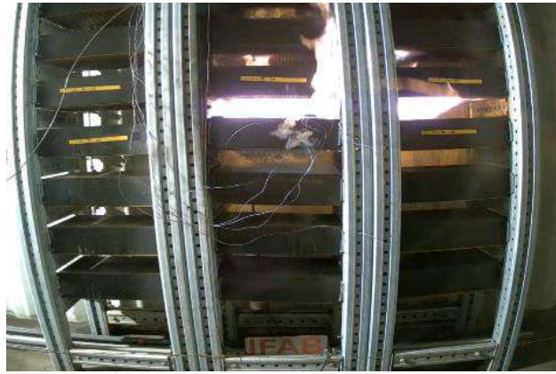
LIB rack within the 20' ESS container
